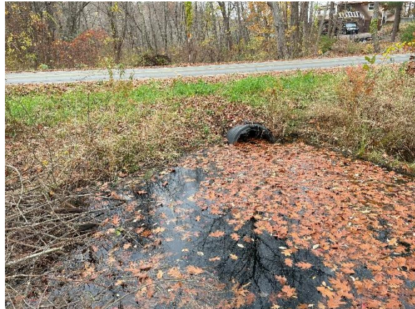
Photo 2: View of upstream culvert inlet, looking west-southwest from the rock wall upstream of Maple Avenue.
