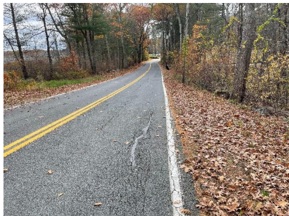
Photo 6: View looking south along Maple Avenue toward the crossing site. The existing culvert is approximately six feet beyond the utility pole on the right side of the photo.
