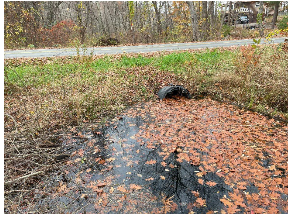
Photo 2: View of upstream culvert inlet, looking west-southwest from the rock wall upstream of Maple Ave.
