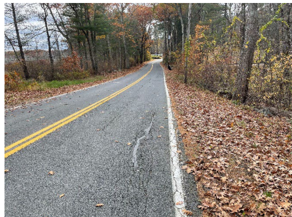
Photo 6: View looking south along Maple Ave toward the crossing site. The existing culvert is approximately six feet beyond the utility pole on the right side of the photo.
